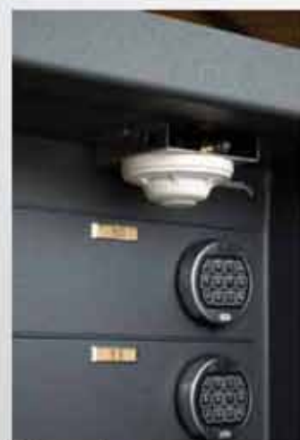
Thermal sensors and door contact
